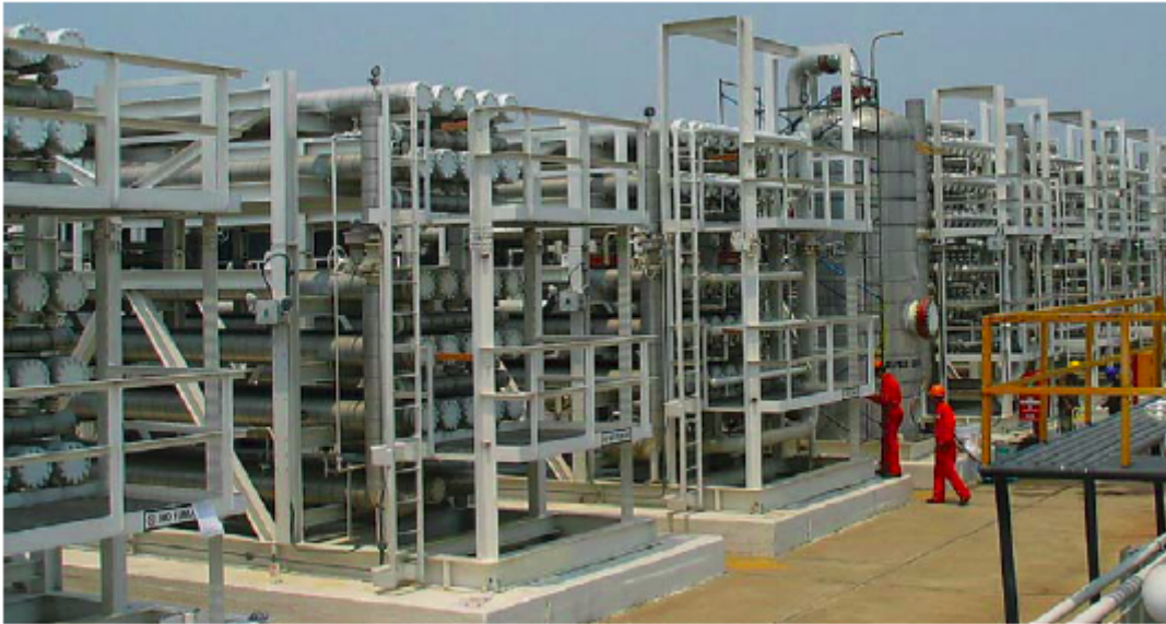
Figure 3 – Separex membrane skids installed at an EOR project in Latin America 6 .
