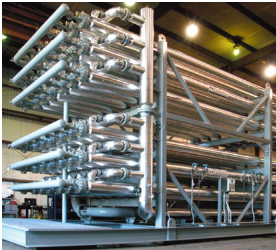
Figure 4 – ProSep membrane skid for CO 2 removal installed in Texas.
