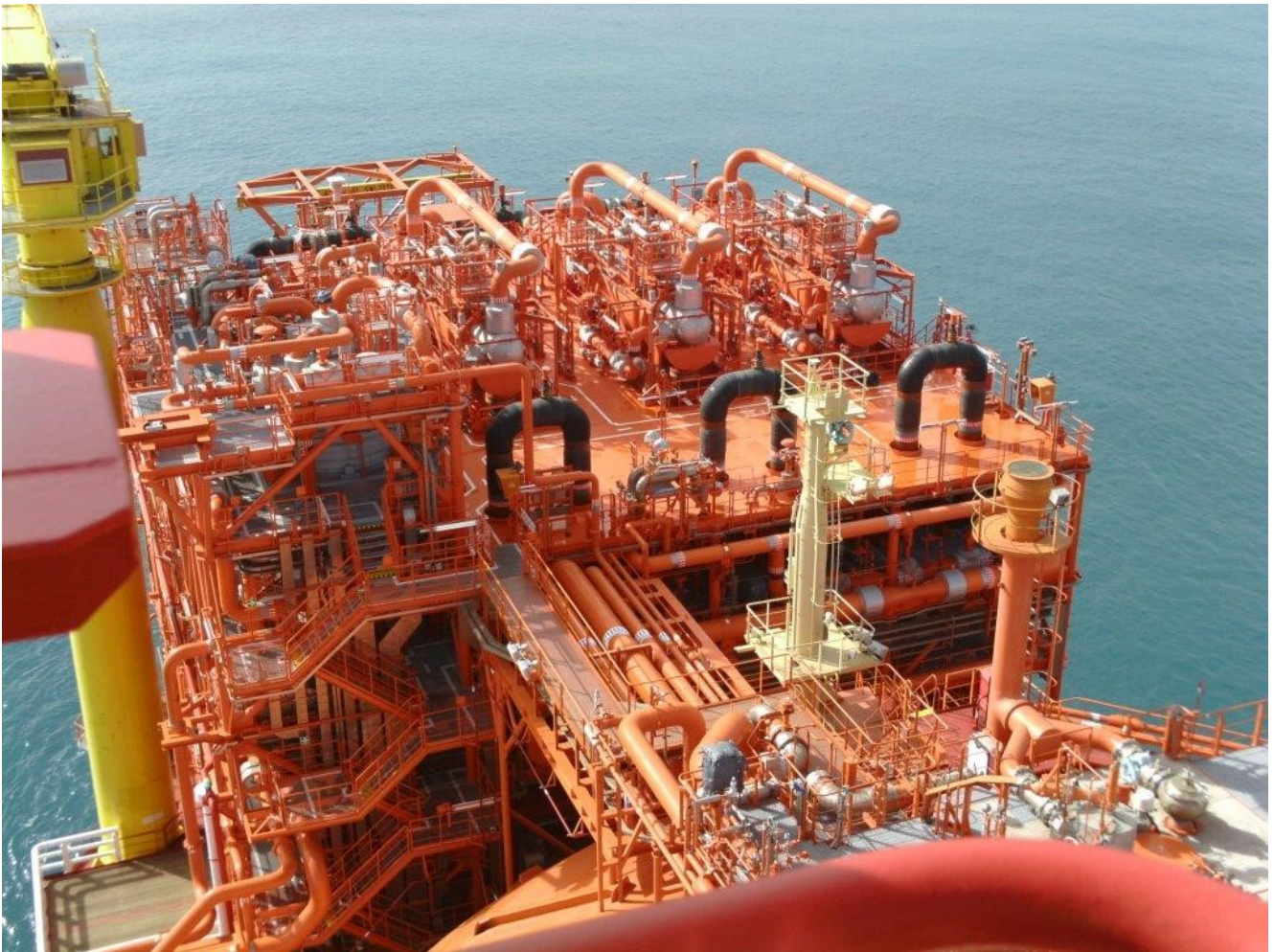
Open Rack Vaporizer Installation on FSRU
