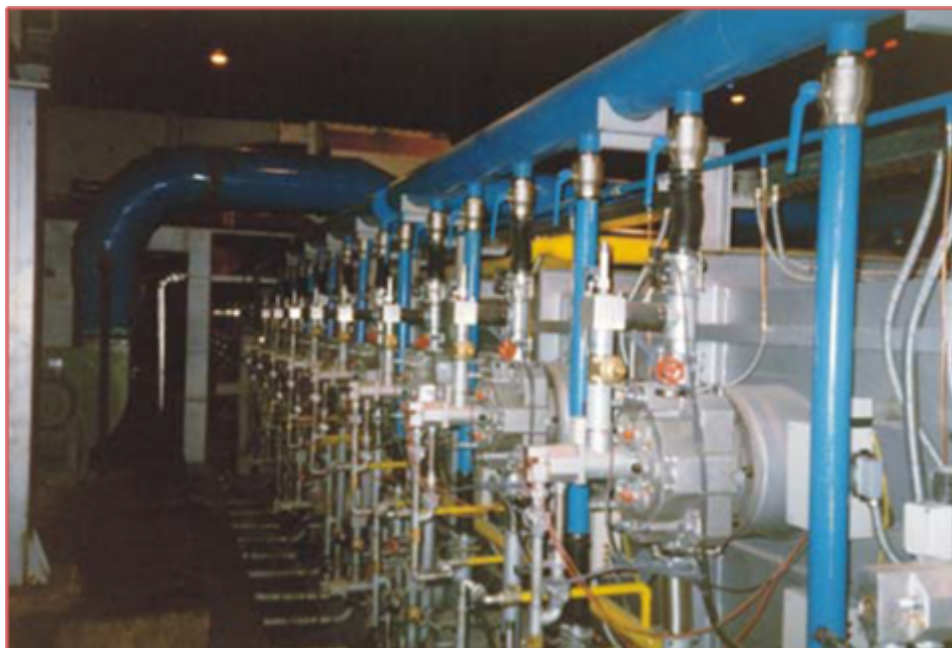
Figure 6 – Regenerative burners in an annealing and pickling line installed at Terni (11)
