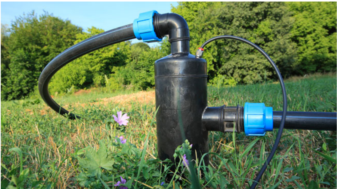
Fig. 4 – EKRT electrode installed on-site
